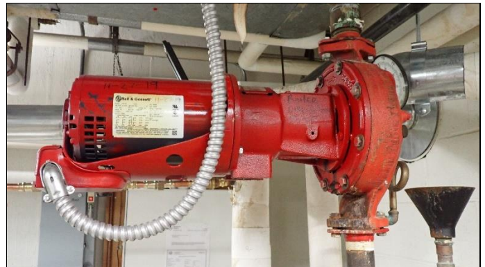
Overview of mechanical equipment
