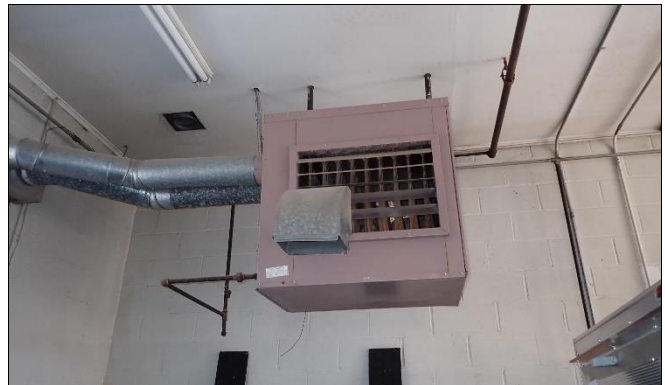
Overview of mechanical equipment
