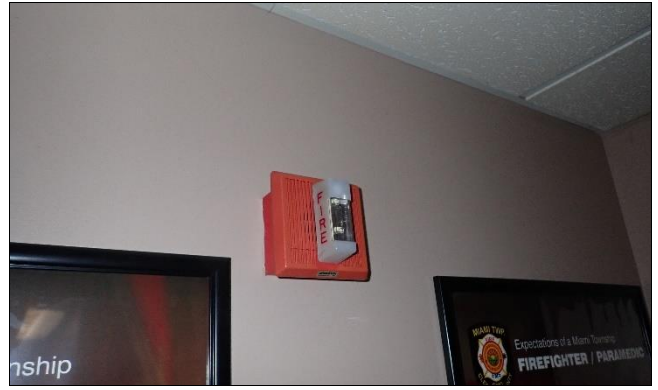
Fire alarm strobe
