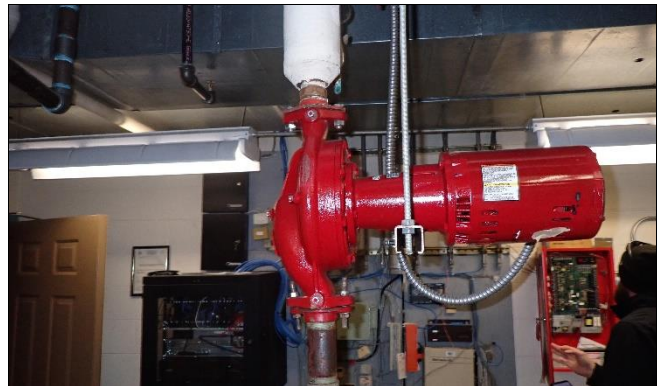
Overview of mechanical equipment
