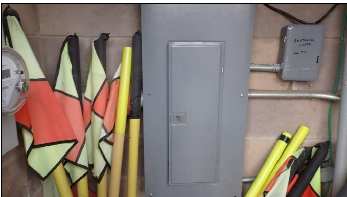
Overview of electrical distribution equipment
