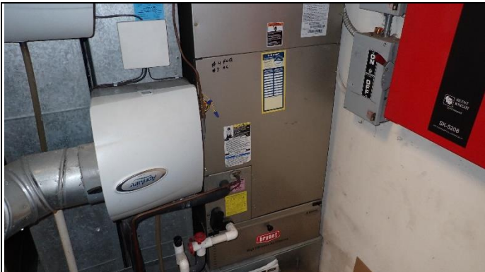
Overview of mechanical equipment
