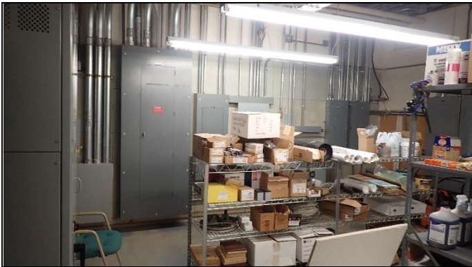
Overview of electrical distribution equipment
