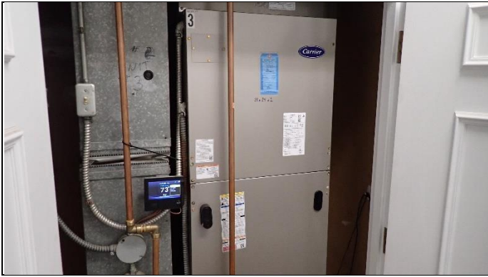
Overview of mechanical equipment
