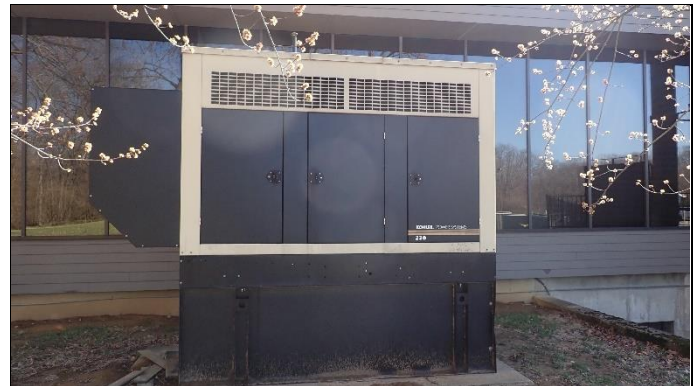
Overview of electrical distribution equipment
