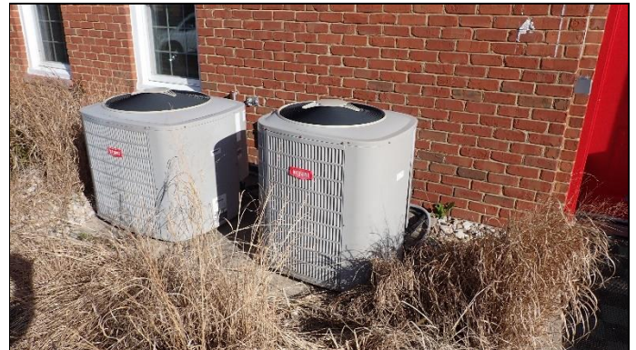
Overview of mechanical equipment
