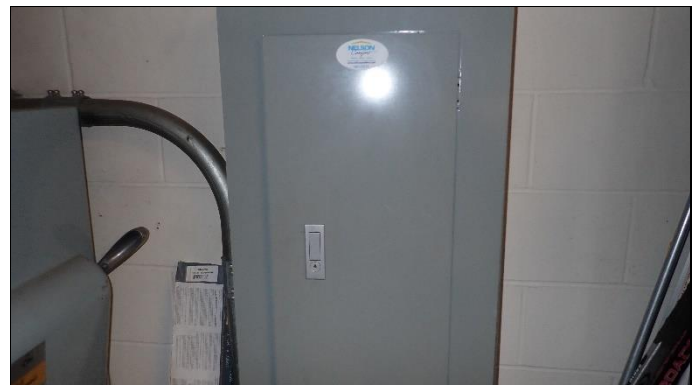
Overview of electrical distribution equipment
