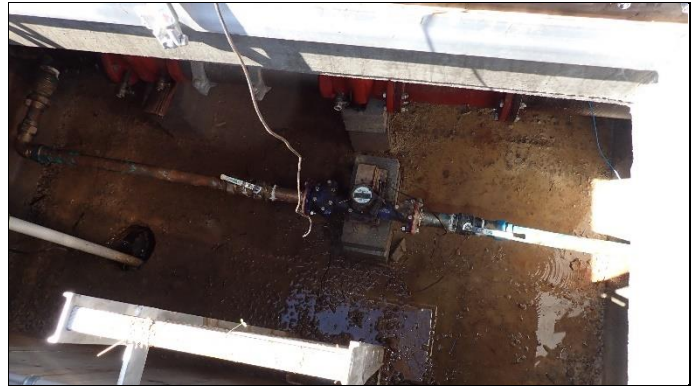
Domestic service entrance
