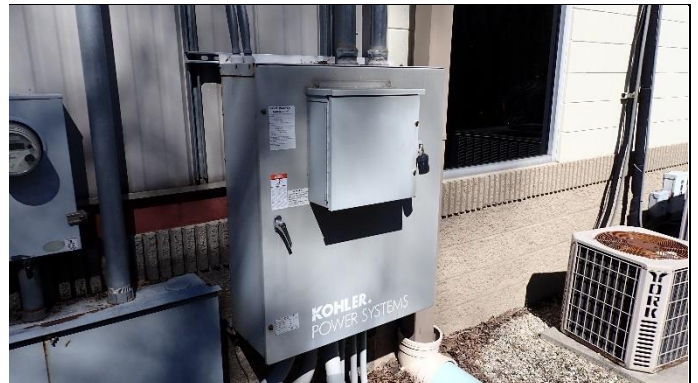
Overview electrical distribution equipment
