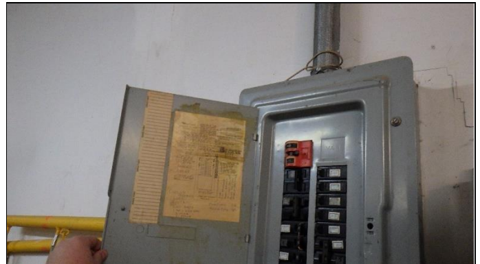
Electrical distribution equipment
