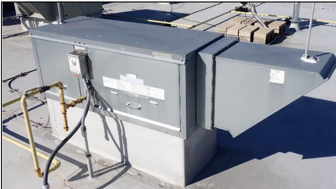
Overview of mechanical equipment
