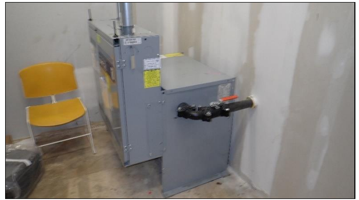
Overview of mechanical equipment
