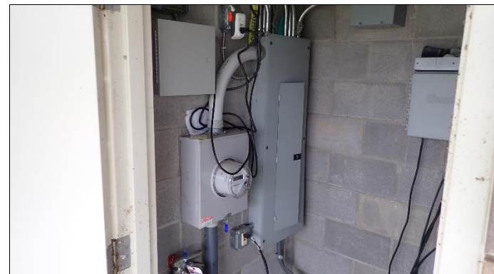
Overview of electrical distribution equipment
