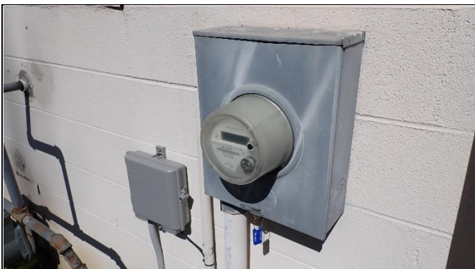
Overview of electrical distribution equipment
