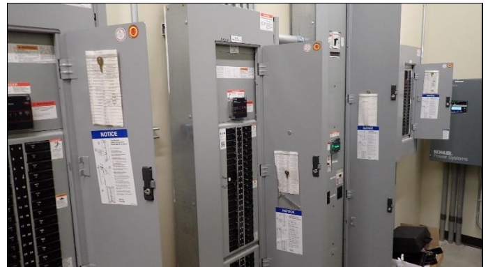
Overview of electrical distribution equipment
