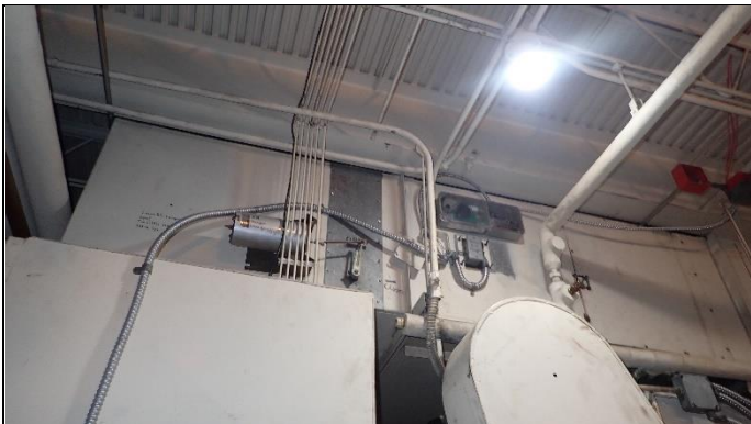
Overview of mechanical equipment
