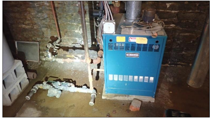
Overview of mechanical equipment
