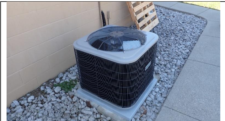
Overview of mechanical equipment
