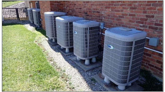
Overview of mechanical equipment
