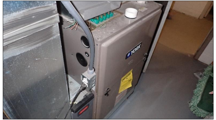
Overview of mechanical equipment
