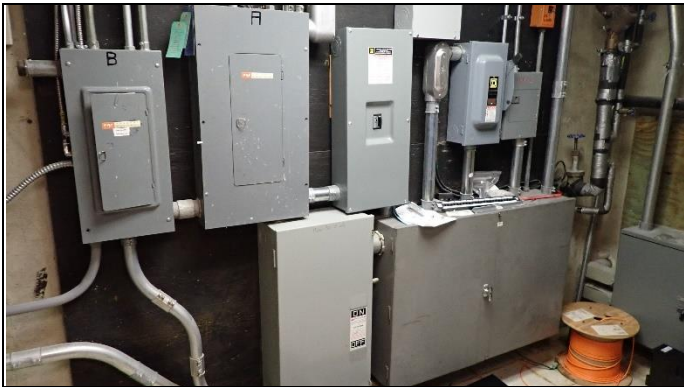
Overview of electrical distribution equipment
