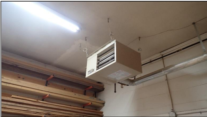
Overview of mechanical equipment
