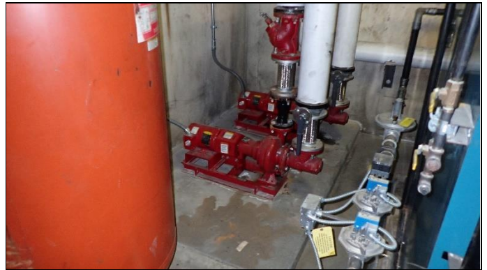
Overview of mechanical equipment
