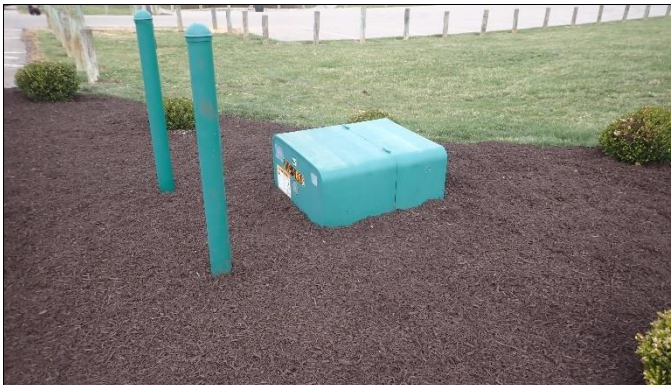
Overview of electrical distribution equipment
