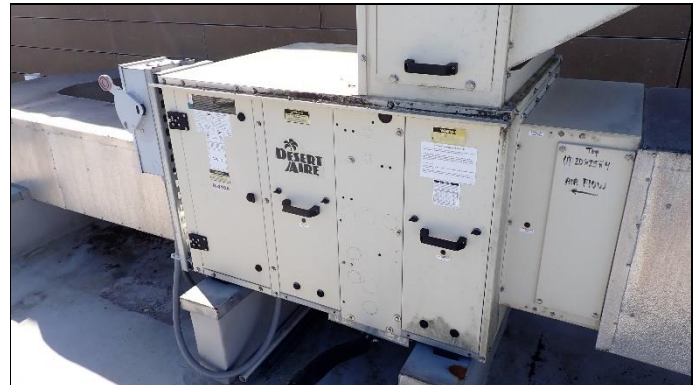
Overview of mechanical equipment
