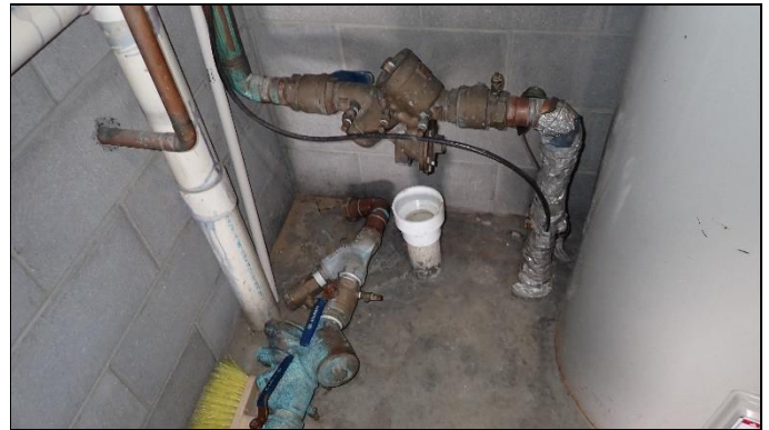
Backflow prevention valve
