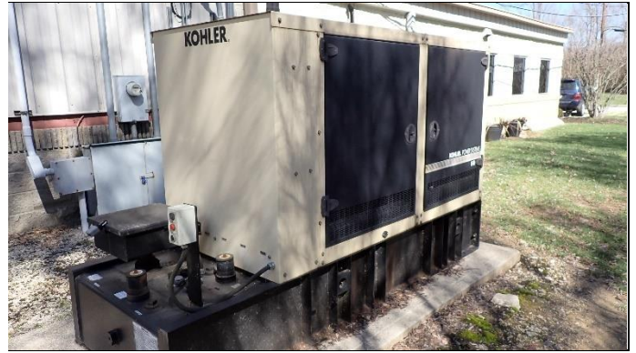
Overview electrical distribution equipment
