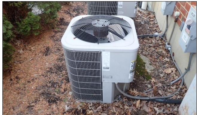
Overview of mechanical equipment
