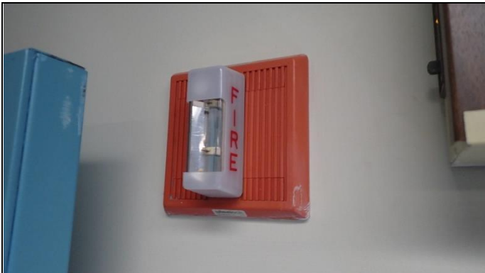
Fire alarm strobe
