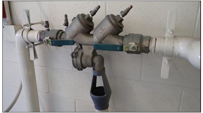
Backflow prevention valve
