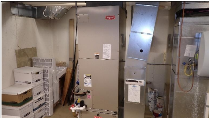
Overview of mechanical equipment
