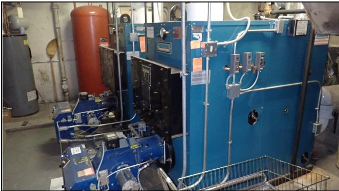
Overview of mechanical equipment
