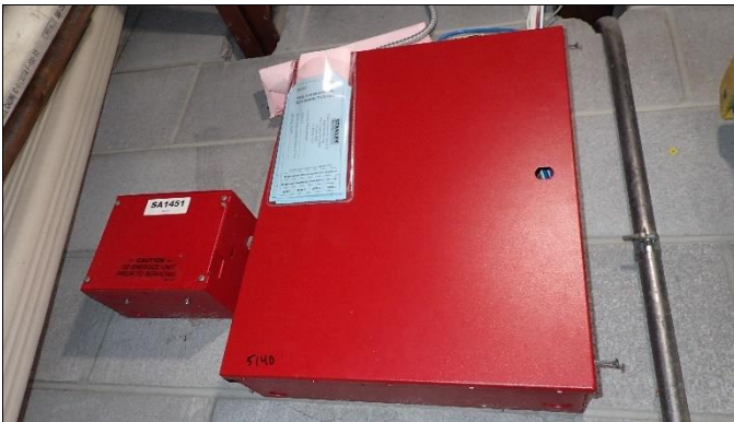
Fire alarm control panel
