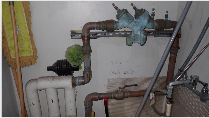
Backflow prevention valve
