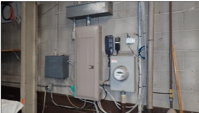
Overview of electrical distribution equipment
