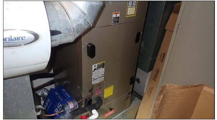
Overview of mechanical equipment
