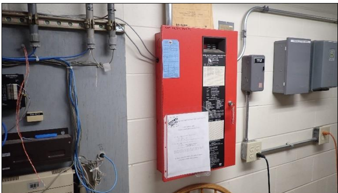
Fire alarm panel
