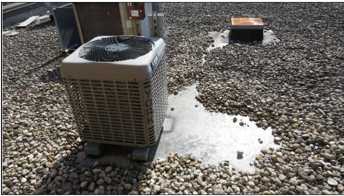
Overview of mechanical equipment
