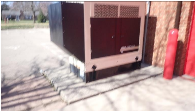
Overview of electrical distribution equipment
