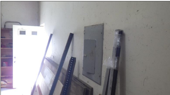
Electrical distribution equipment
