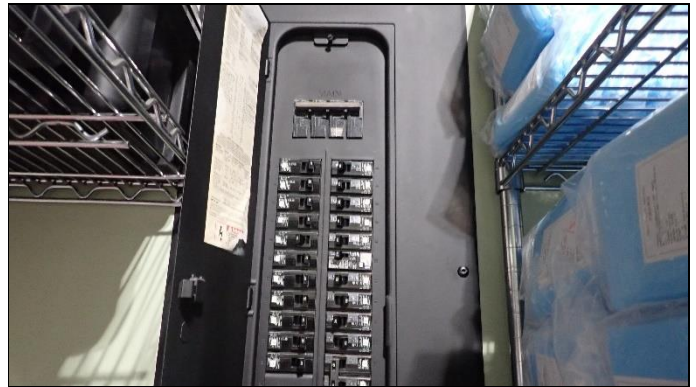
Overview of electrical distribution equipment
