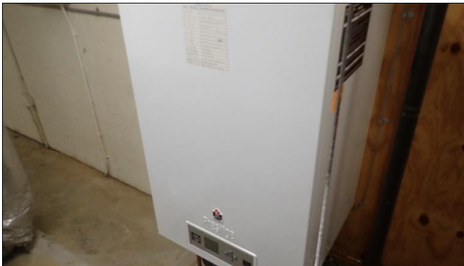
Overview of mechanical equipment
