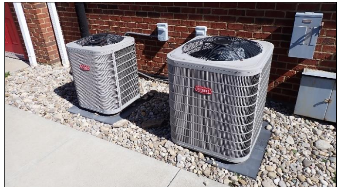
Overview of mechanical equipment
