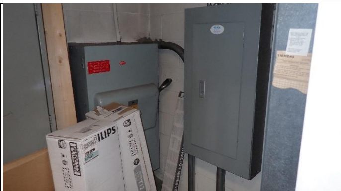
Overview of electrical distribution equipment
