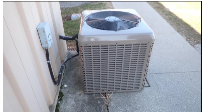
Overview of mechanical equipment
