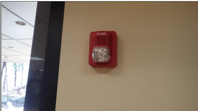
Fire alarm strobe
