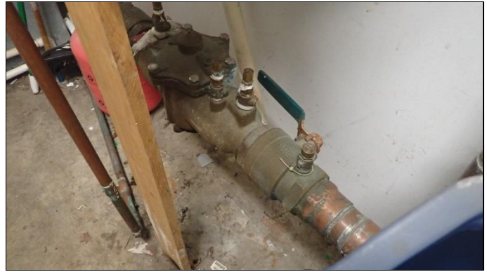
Backflow prevention valve
