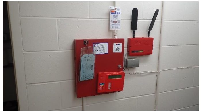
Fire alarm control panel
