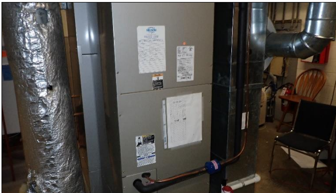
Overview of mechanical equipment
