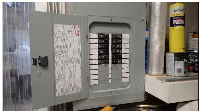
Overview of electrical distribution equipment
