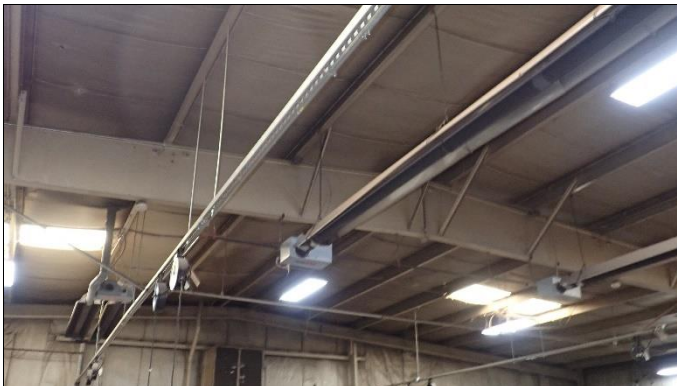
Overview of mechanical equipment
