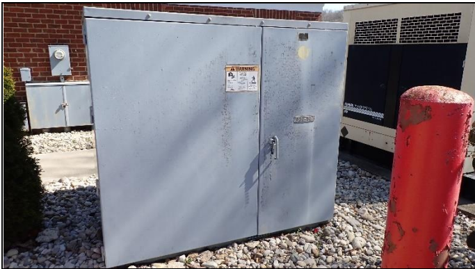
Overview of electrical distribution equipment
