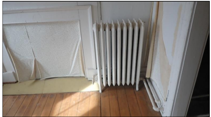
Overview of mechanical equipment
