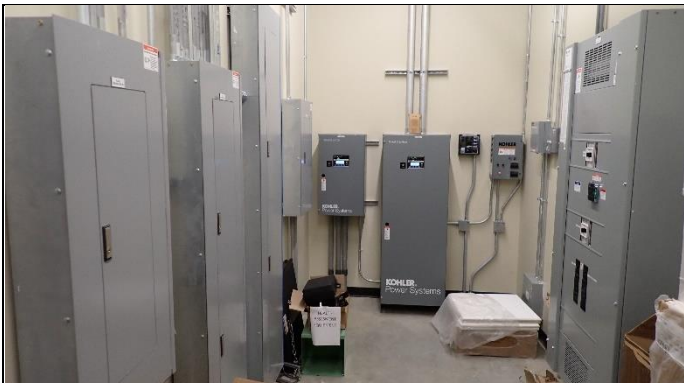
Overview of electrical distribution equipment
