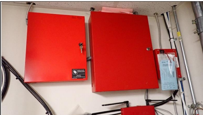
Fire alarm panel
