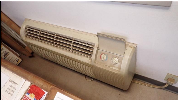
Overview of mechanical equipment
