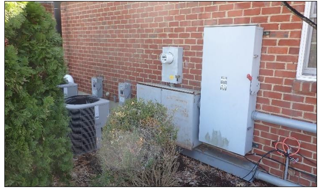
Overview of electrical distribution equipment
