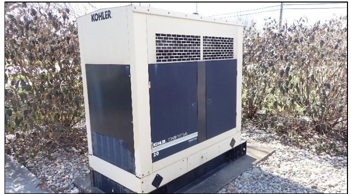
Overview of electrical distribution equipment
