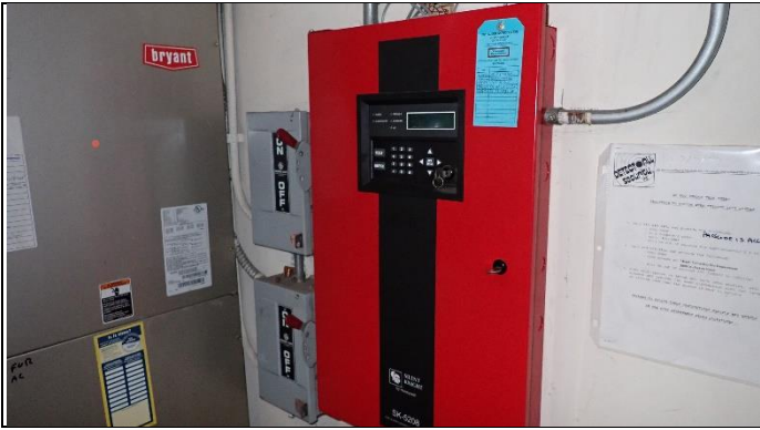
Fire alarm panel
