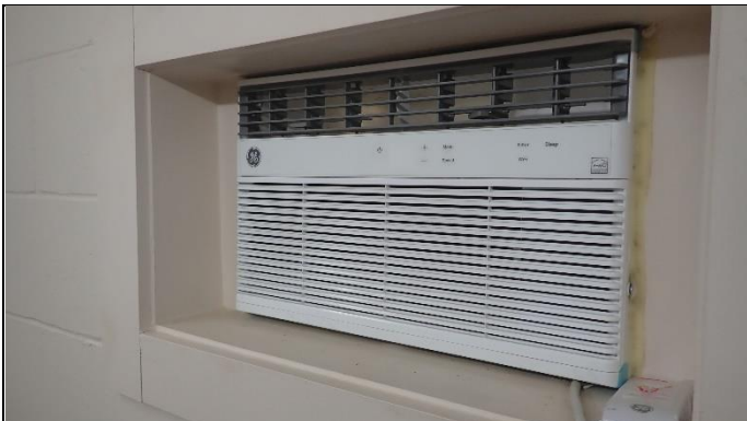
Overview of mechanical equipment
