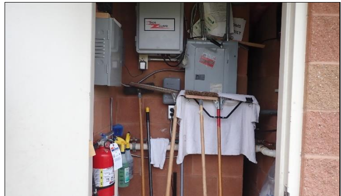
Overview of electrical distribution equipment
