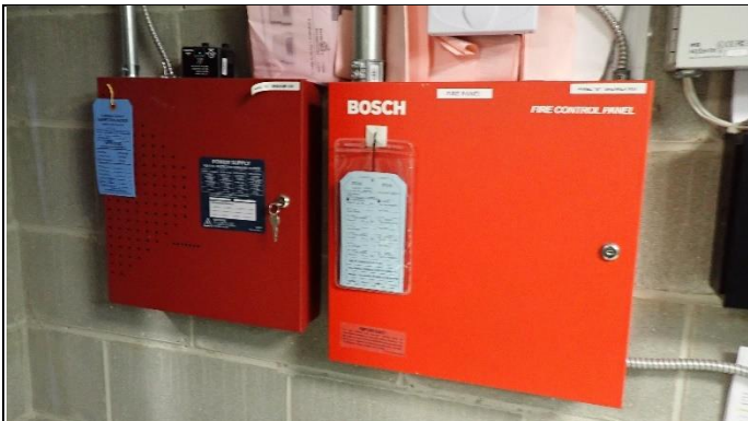
Fire alarm panel
