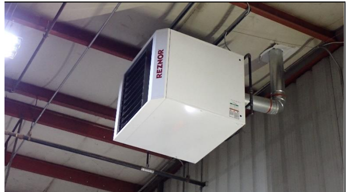
Overview of mechanical equipment
