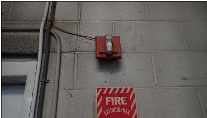
Fire alarm strobe
