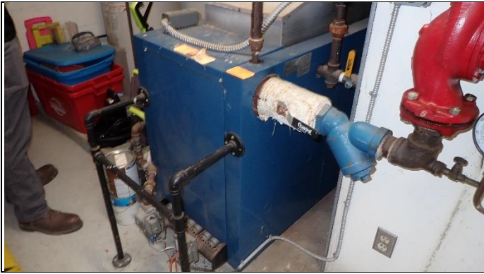
Overview of mechanical equipment
