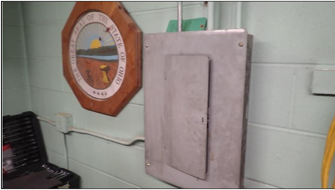
Electrical distribution equipment
