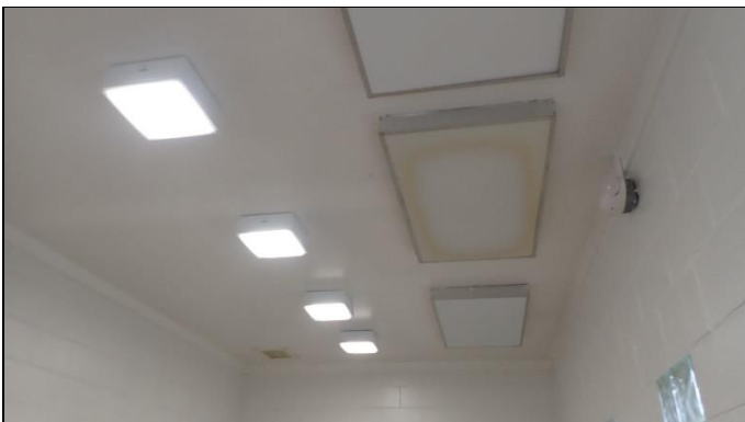
Overview of mechanical equipment
