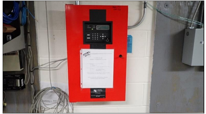
Fire alarm panel
