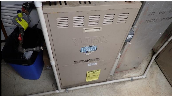
Overview of mechanical equipment
