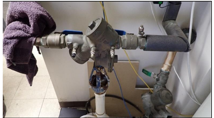
Backflow prevention valve
