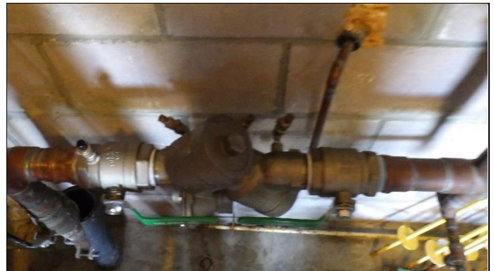
Backflow prevention valve
