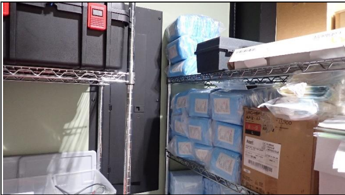
Overview of electrical distribution equipment
