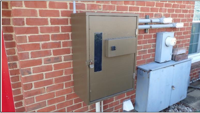
Overview of electrical distribution equipment
