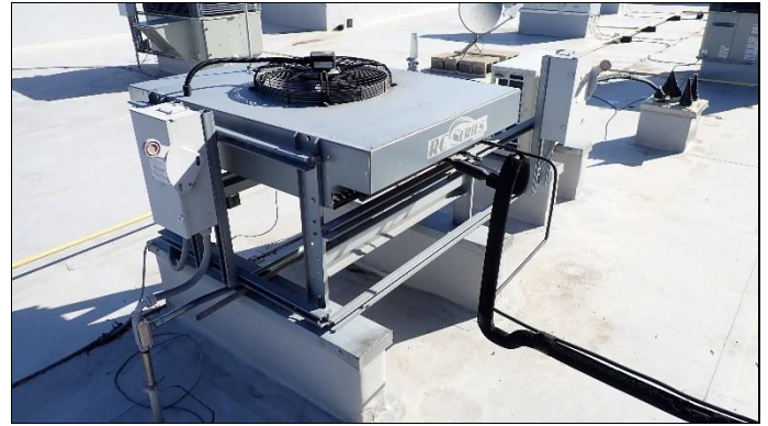
Overview of mechanical equipment
