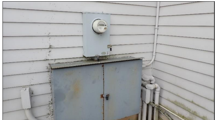
Electrical distribution equipment
