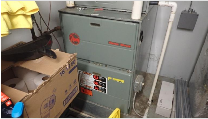
Overview of mechanical equipment
