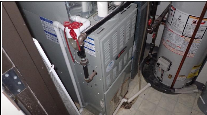
Overview of mechanical equipment
