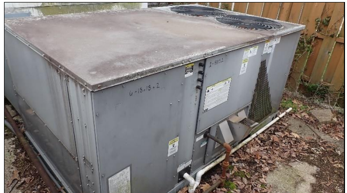
Overview of mechanical equipment
