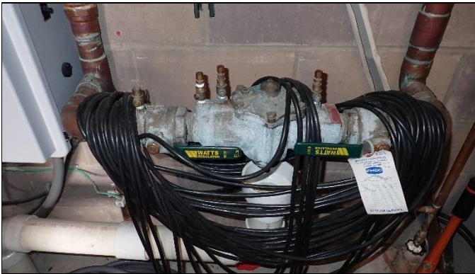
Backflow prevention valve
