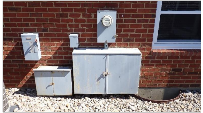
Overview of electrical distribution equipment
