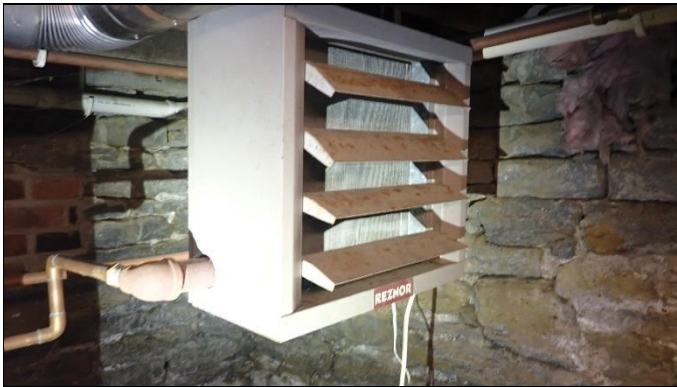
Overview of mechanical equipment
