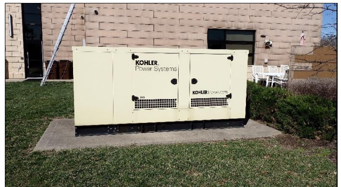
Overview of electrical distribution equipment
