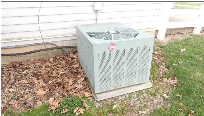
Overview of mechanical equipment
