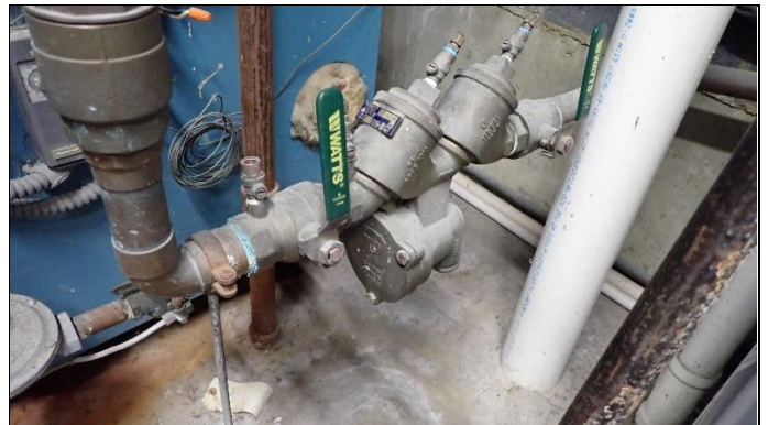
Backflow prevention valve
