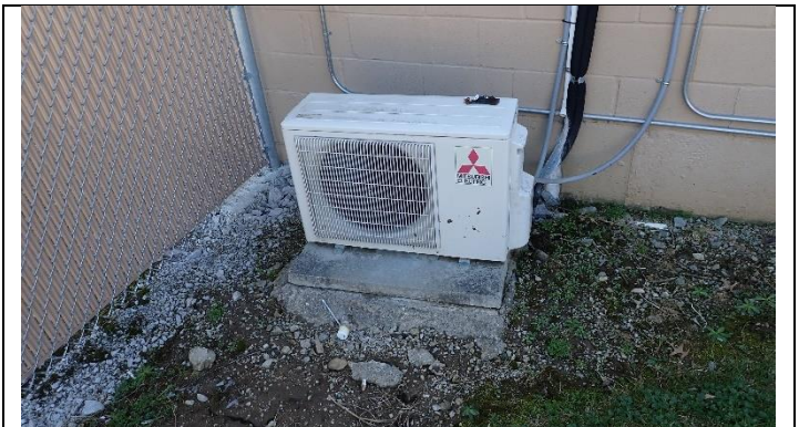
Overview of mechanical equipment
