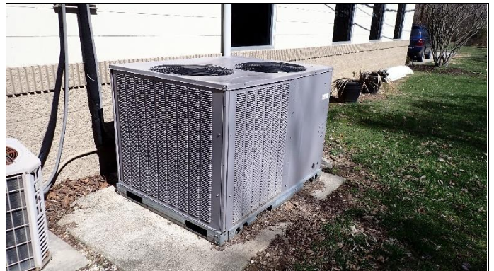
Overview of mechanical equipment
