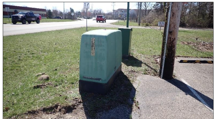
Overview of electrical distribution equipment
