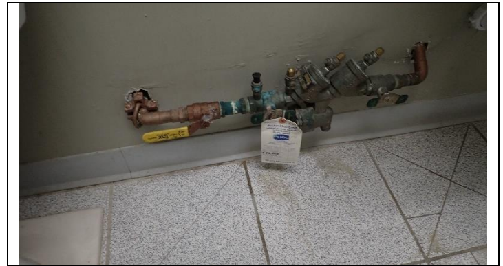
Backflow prevention valve
