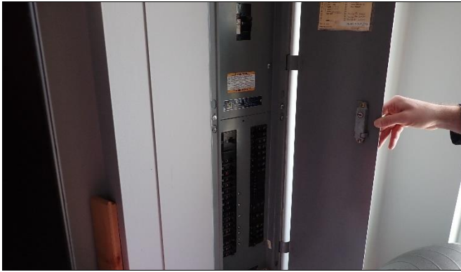
Electrical distribution equipment
