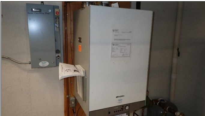
Overview of mechanical equipment
