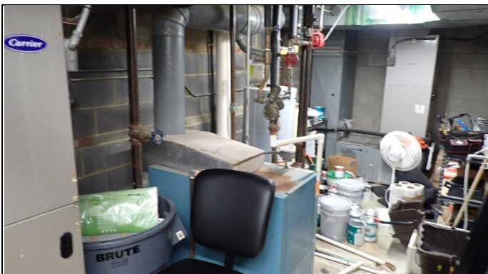
Overview of mechanical equipment
