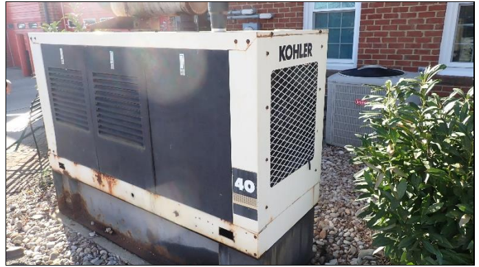
Overview of electrical distribution equipment
