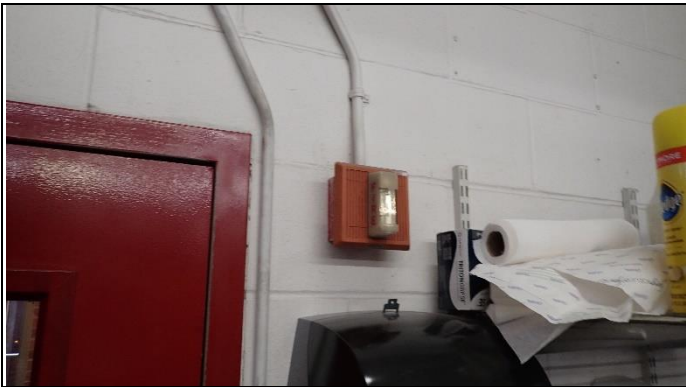
Fire alarm strobe
