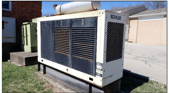
Overview of electrical distribution equipment
