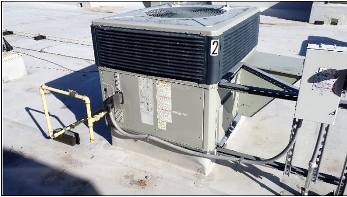
Overview of mechanical equipment
