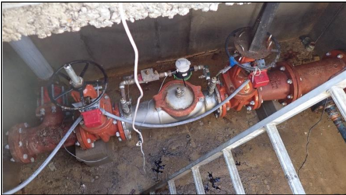
Heavy duty backflow valve at service entrance
