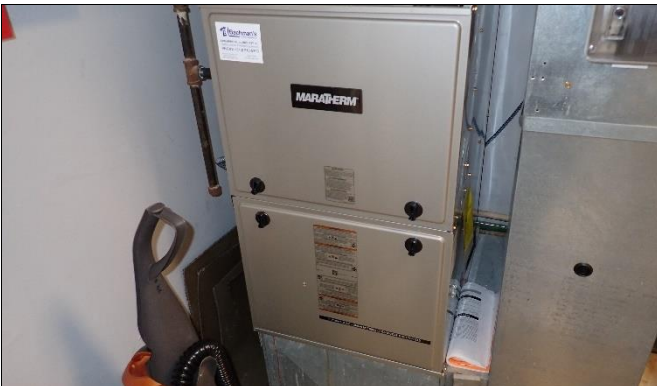
Overview of mechanical equipment
