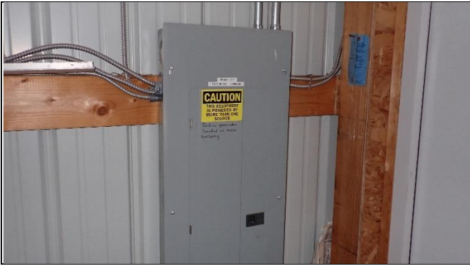
Overview electrical distribution equipment
