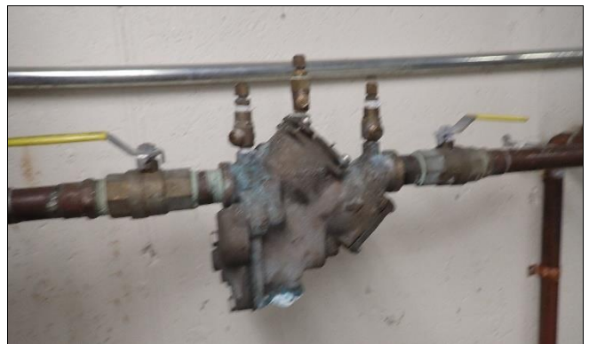
Backflow prevention valve
