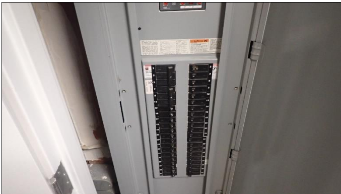
Electrical distribution equipment
