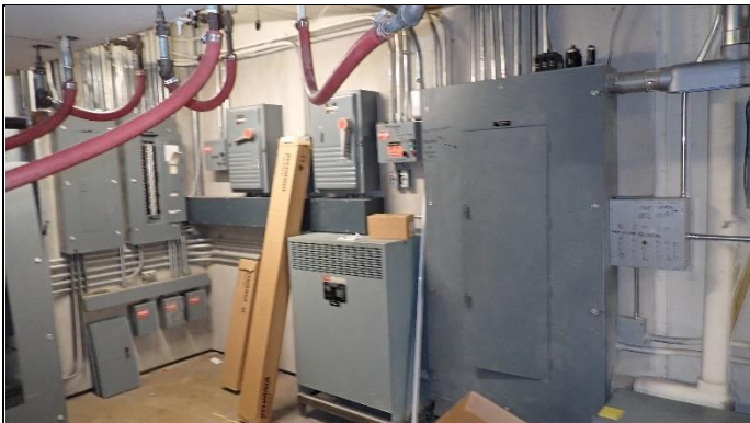
Overview of electrical distribution equipment
