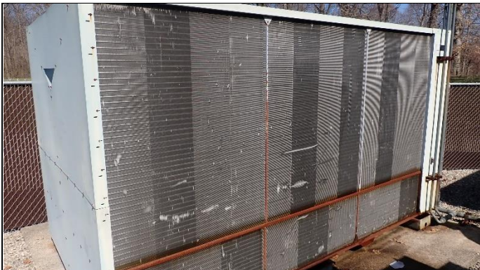
Overview of mechanical equipment
