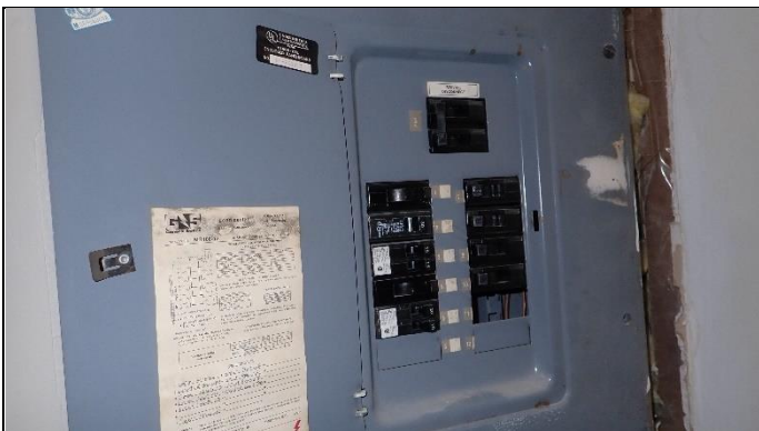
Overview of electrical distribution equipment
