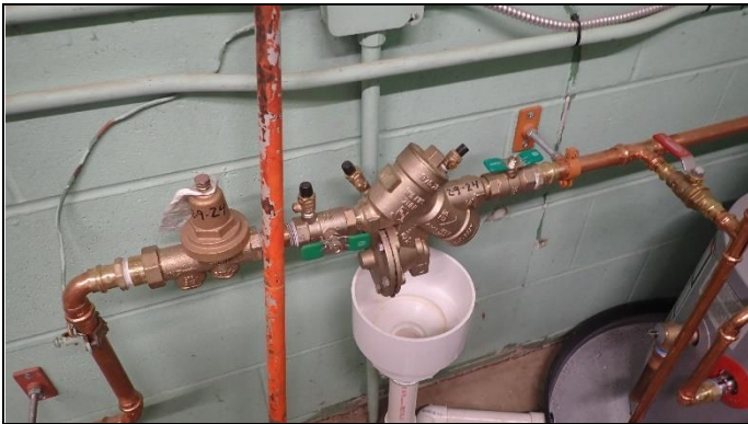
Backflow prevention valve
