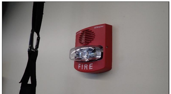
Fire alarm strobe
