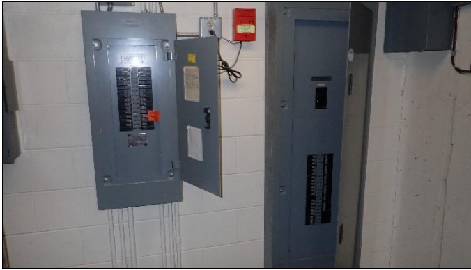
Overview of electrical distribution equipment
