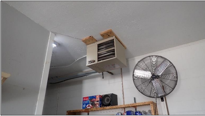
Overview of mechanical equipment
