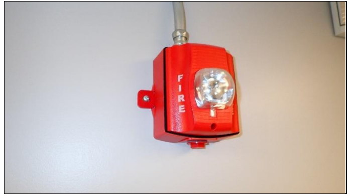
Fire alarm strobe
