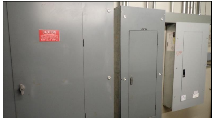
Overview of electrical distribution equipment
