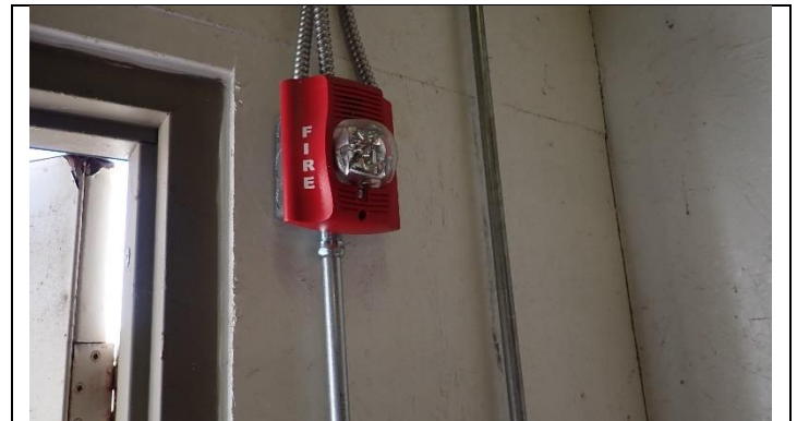
Fire alarm strobe
