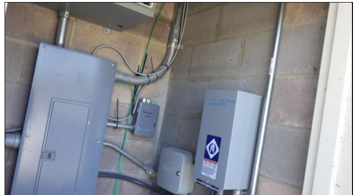
Electrical distribution equipment
