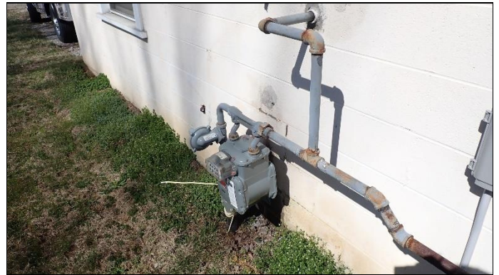
Overview of mechanical equipment
