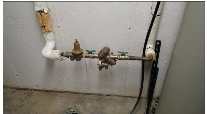
Backflow prevention valve
