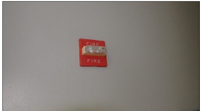
Fire alarm strobe
