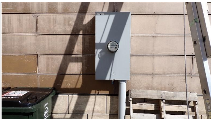
Overview of electrical distribution equipment
