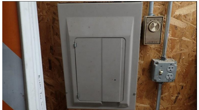
Overview of electrical distribution equipment
