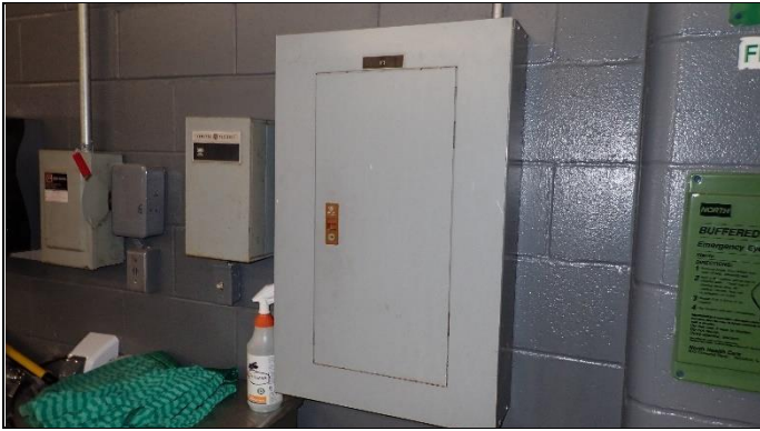
Overview of electrical distribution equipment
