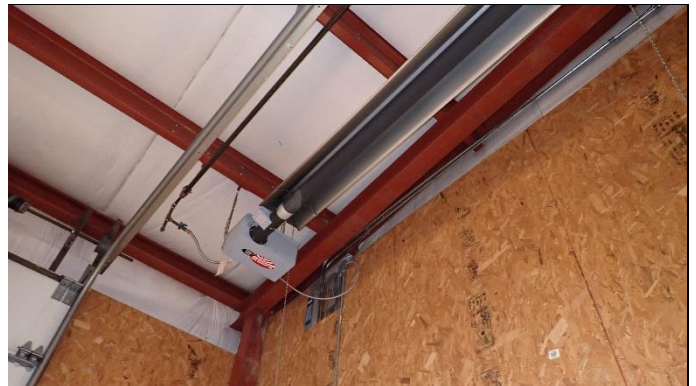
Overview of mechanical equipment
