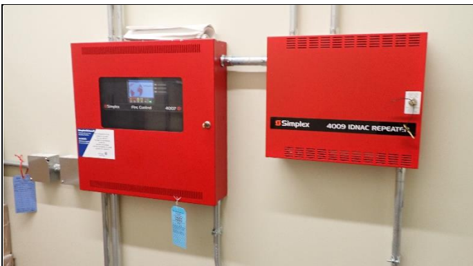
Fire alarm control panel
