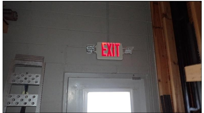
Emergency lighting and signage
