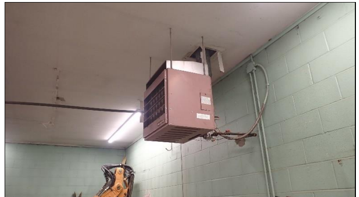
Overview of mechanical equipment
