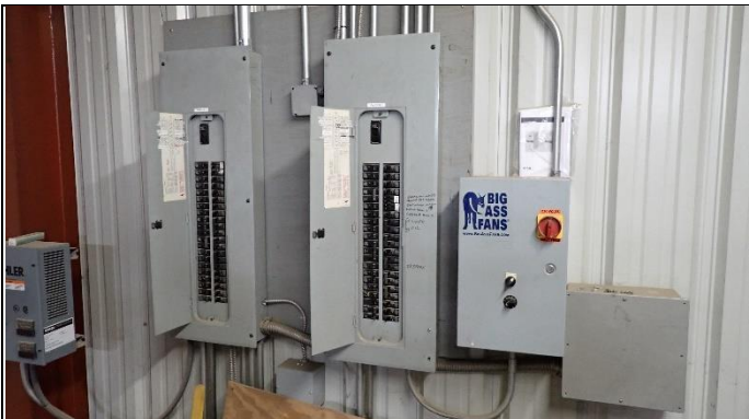
Overview electrical distribution equipment
